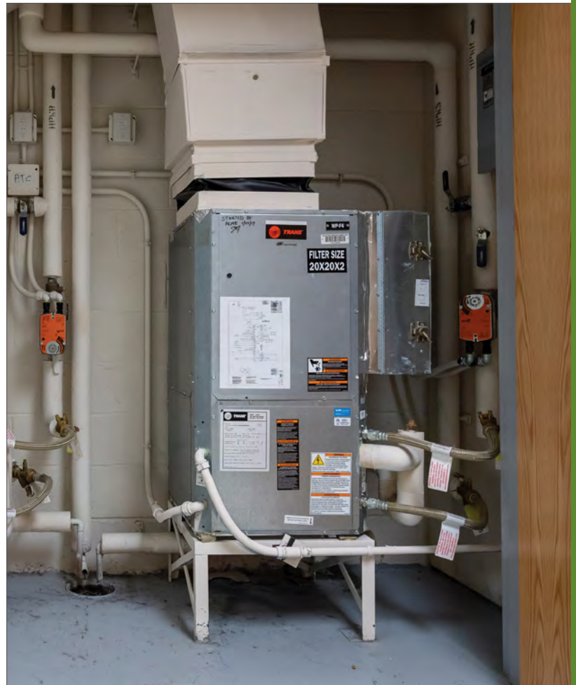
Ground Source Heat Pumps heat and cool using the constant temperature of the earth extracted from wells hundreds of feet deep for the source of heat transfer.
