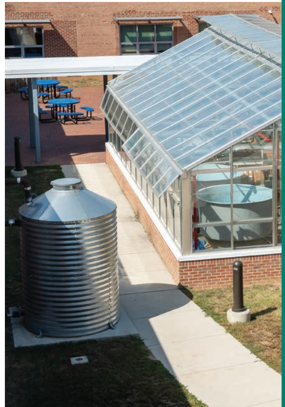
Roof rainwater storage container for watering plants in the greenhouse at Thomas Jefferson High School for Science and Technology.
